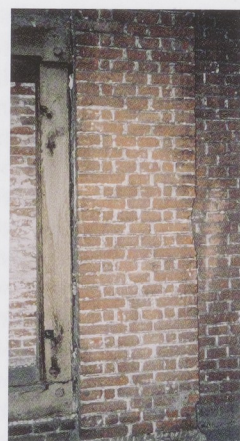
Fig. 16 Original window frame of the exterior wall of the first floor of the Kloveniers- doelen, found during renovation work at the Hotel Doelen during the 1970s.
