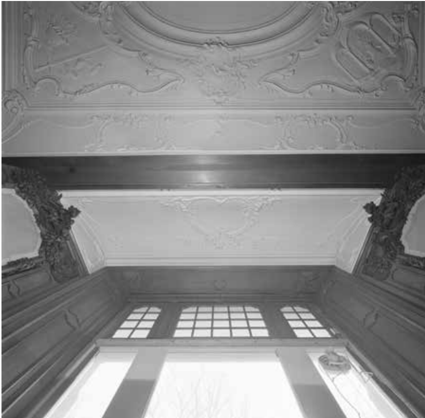
Fig. 8 ANONYMOUS, Bay with Existing Window and a Partially New Plaster Ceiling with Matching Decoration, 1976. Photograph. Amsterdam, Amsterdam Museum Archives, Dismantlement logbook.
